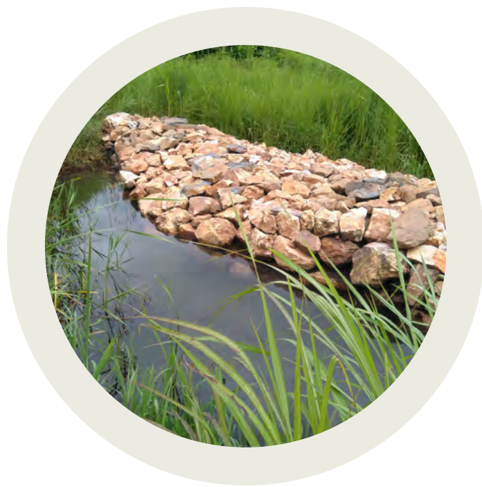
Leaky weir for enhanced water infiltration in the Kafue River catchment area, Zambia. © NIRAS
